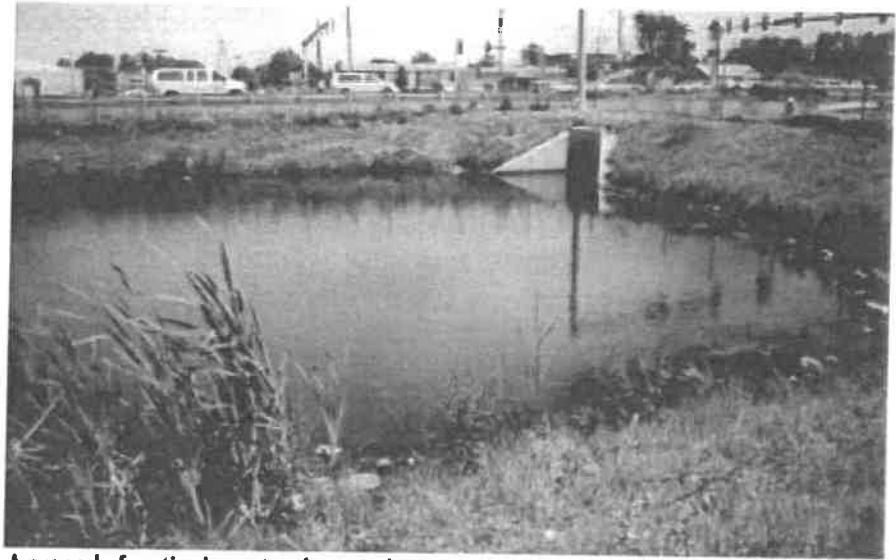
A properly functioning retention pond.
